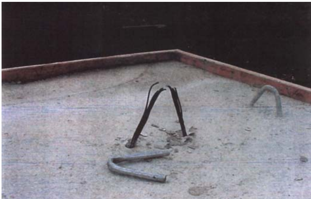
Photo 6. Pulling iron strand failure
